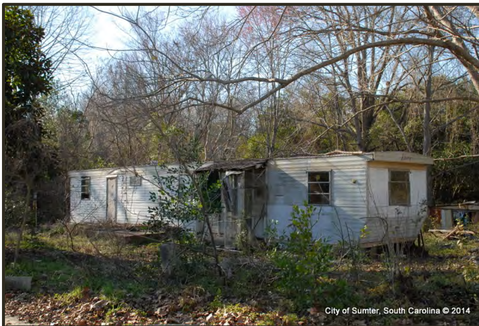
Photograph 76 Wilder Example of "Hazard" Condition Property
