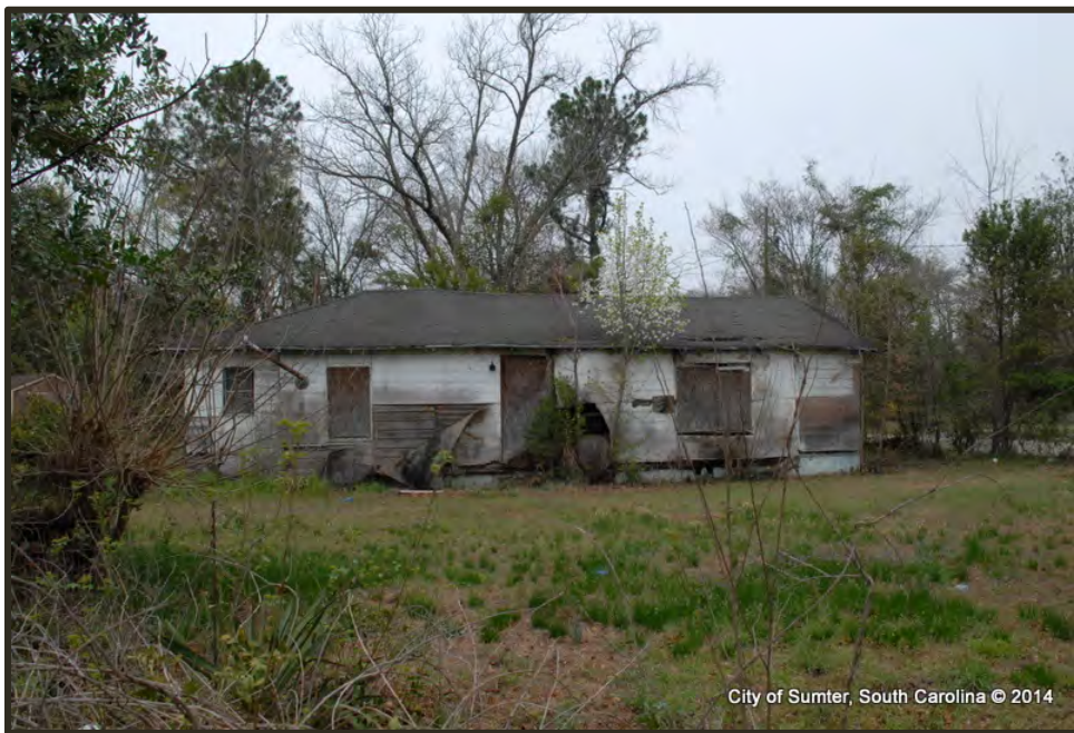
Photograph 4 Bates Example of "Hazard" Condition Property
