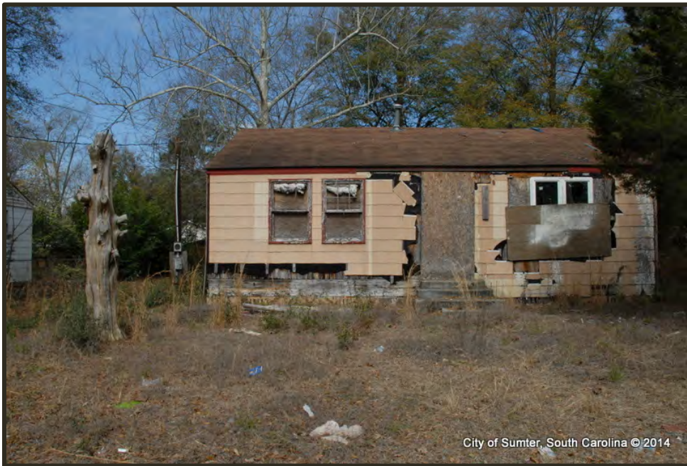
Photograph 72 Swan Lake Example of "Hazard" Condition Property
