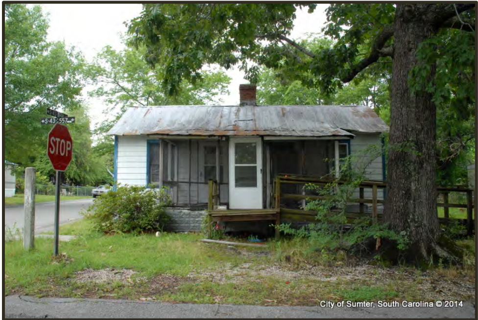
Photograph 30 Loring Example of "Hazard" Condition Property
