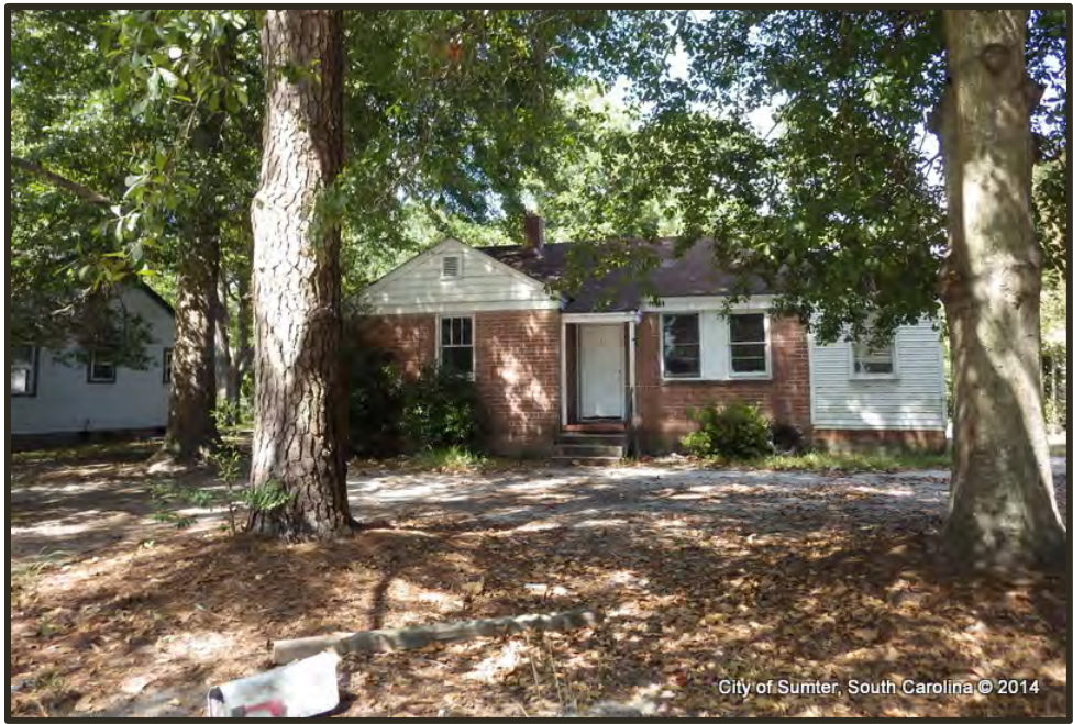
Photograph 17 Folsom Park Example of "Poor" Condition Property
