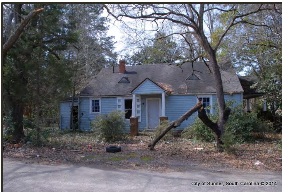
Photograph 40 Morris College Example of "Hazard" Condition Property
