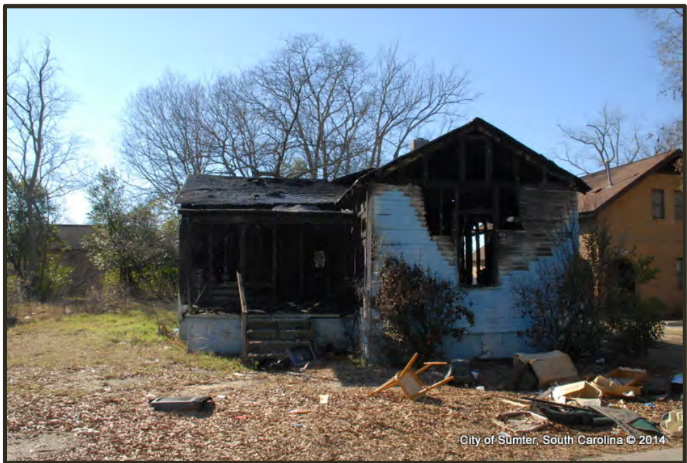
Photograph 52 Savage Glover Example of "Hazard" Condition Property
