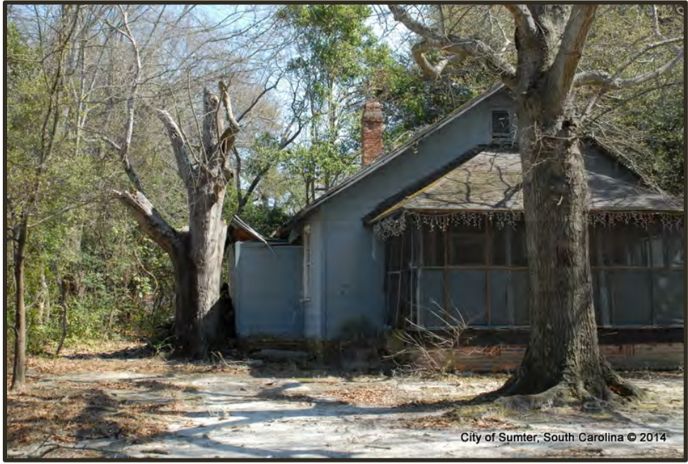
Photograph 18 Folsom Park Example of "Hazard" Condition Property
