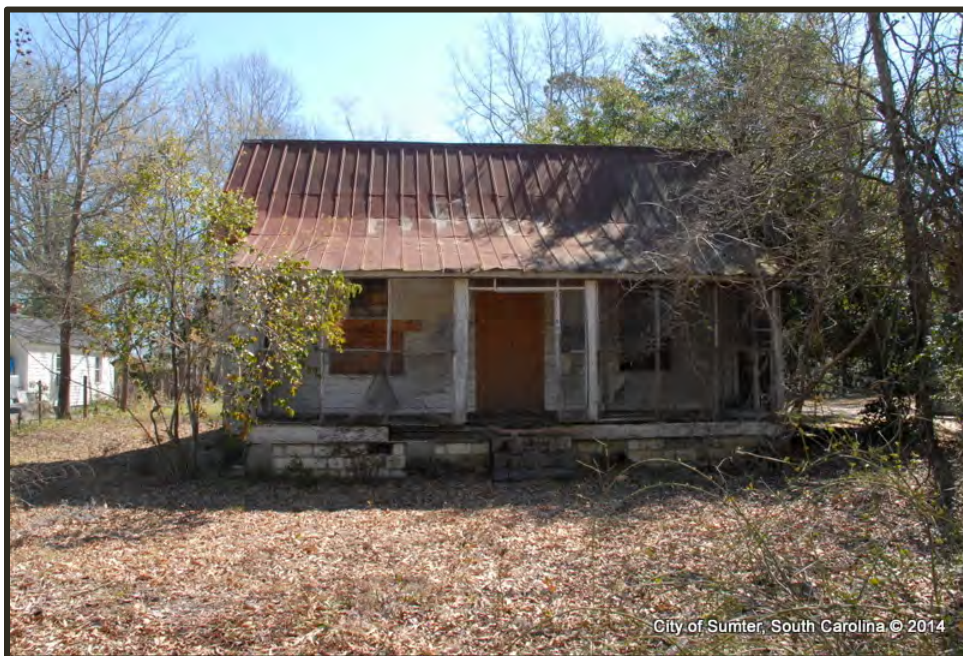
Photograph 14 Crosswell Example of "Hazard" Condition Property
