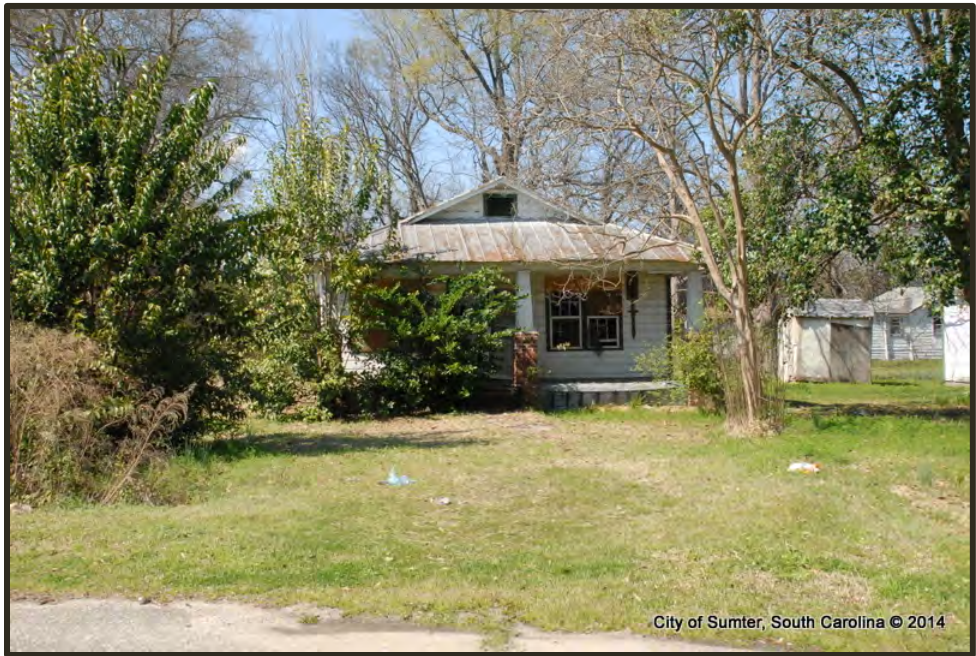
Photograph 33 Magnolia-Harmony Example of "Poor" Condition Property
