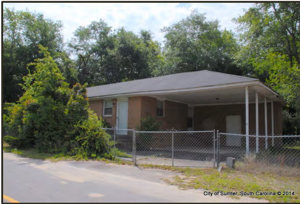
Photograph 75 Wilder Example of "Poor" Condition Property
