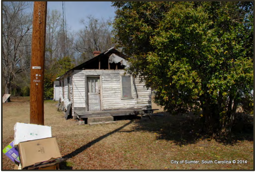
Photograph 48 Palmetto Example of "Hazard" Condition Property
