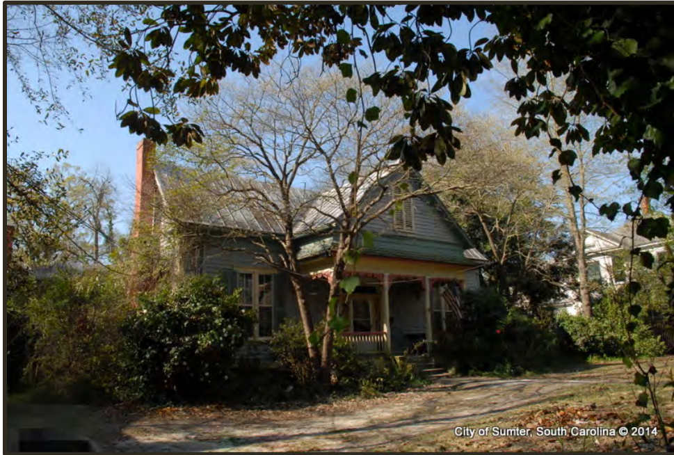
Photograph 21 Hampton Park Example of "Poor" Condition Property
