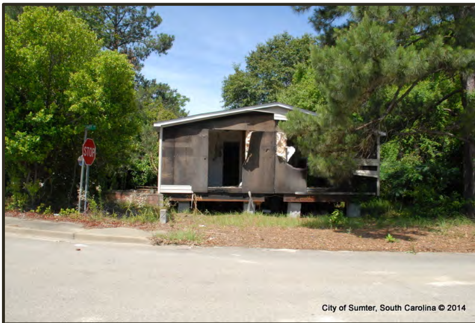
Photograph 64 Spectrum Example of "hazard" Condition Property
