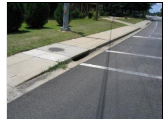
Crosswalk without curb ramp (Pinewood Road)
