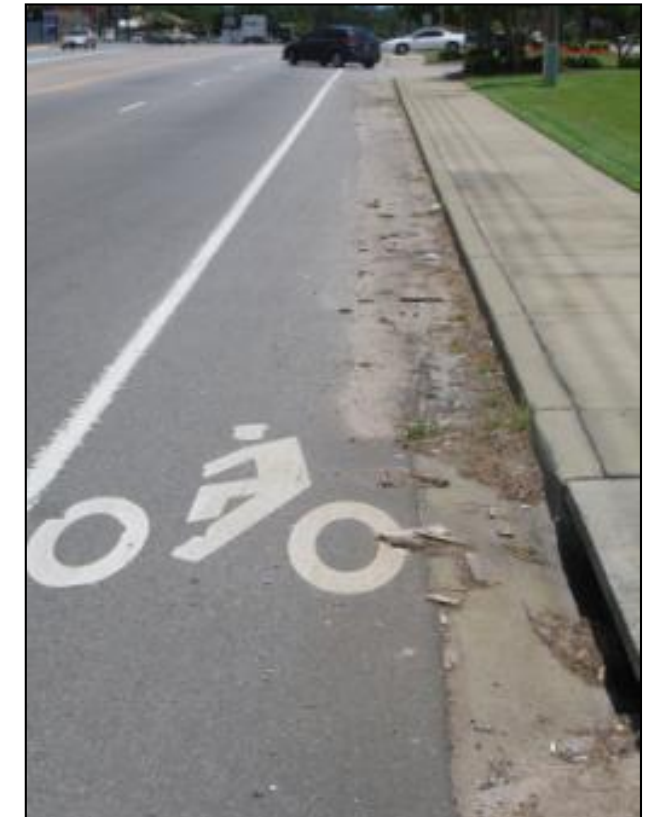
McCrays Mill Road bike lane in need of maintenance
