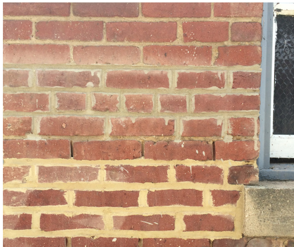
The new mortar does not match the historic mortar in color or tooling.
