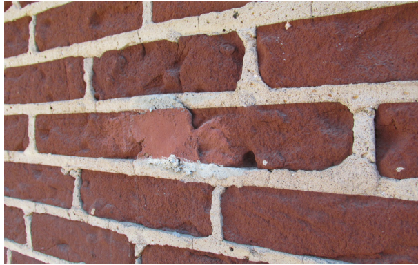
Sandblasting can irreversibly damage masonry.
